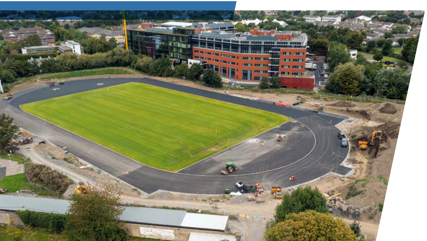
The new UCD Running Track is under construction with planned completion in 2022.
